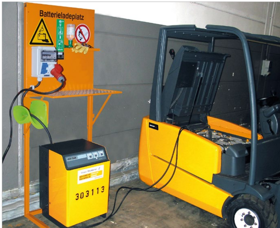
BL with CEEform socket 400 V charging the battery of an electric forklift truck
